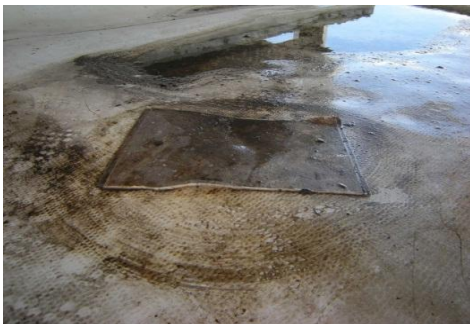
Failing Patch Repair on Roof
