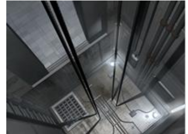
Elevator shaft subject to wind issues
